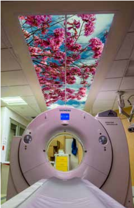
Backlit luminaire at St. Jude Medical Center:
